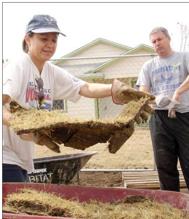
Master Sgt. Toni Abrego (left) and Tech. Sgt. Larry Wright lay sod in the backyard of a Habitat for Humanity home Saturday in San Antonio. Habitat for Humanity seeks volunteers each Saturday throughout the spring and summer to help build and landscape homes for qualified low-income families. For volunteer information, visit www.habitatsa.org . (Photo by Staff Sgt. Jennier Lindsey)
