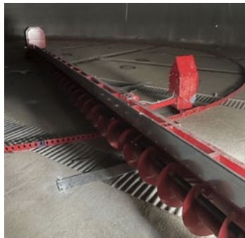
ADM Romania silo modernized with 16 pieces of new grain handling equipment
